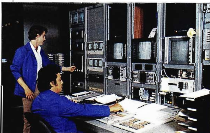
Close-up view of console in Master Control.
