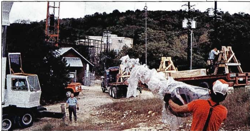
RCA TFU-28DAS high power peanut pattern pylon antenna arrives for installation . . . and is soon mounted atop existing 1290' tower providing KBVO with excellent coverage.
